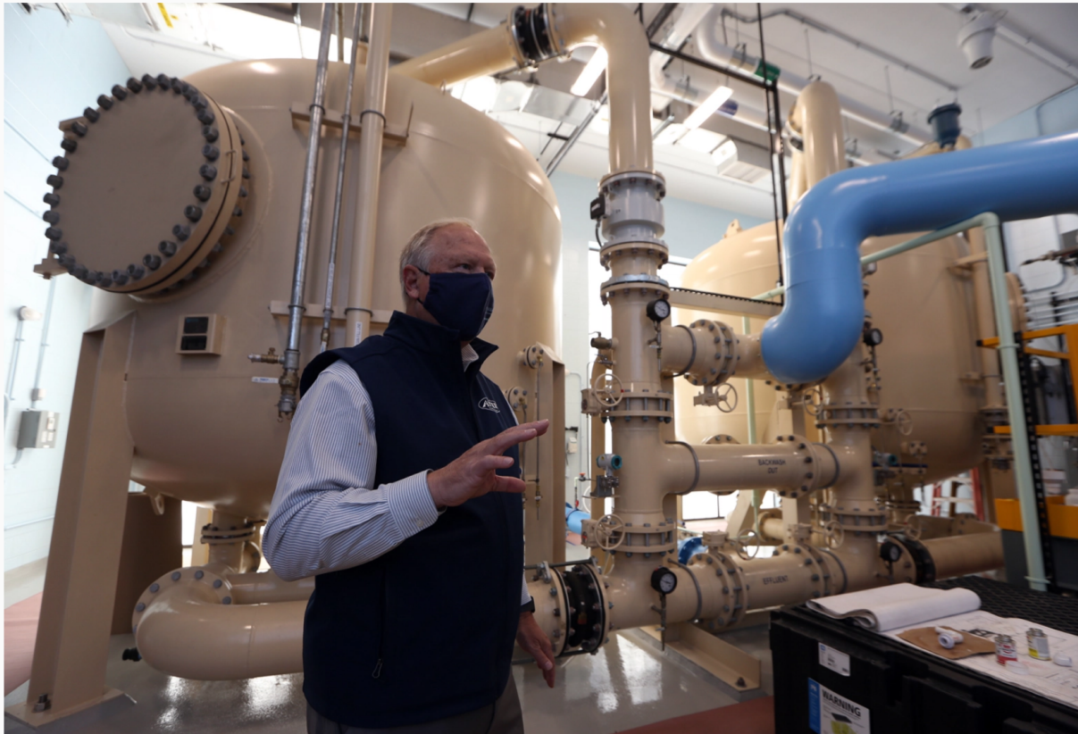
Ayer DPW Superintendent Mark Wetzel gives a tour of the Grove Pond Water Treatment Plant's new wing containing an ionic exchange treatment plant to remove PFAS, the first in Massachusetts. (SUN/Julia Malakie)
